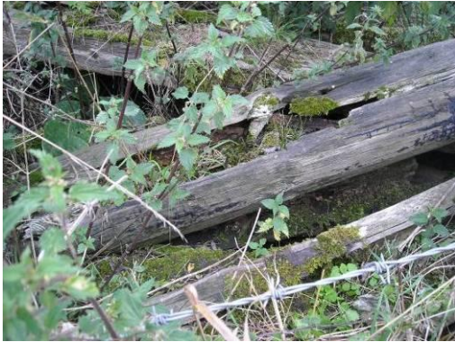
Fig. 16 Partially rotting timbers on ground
